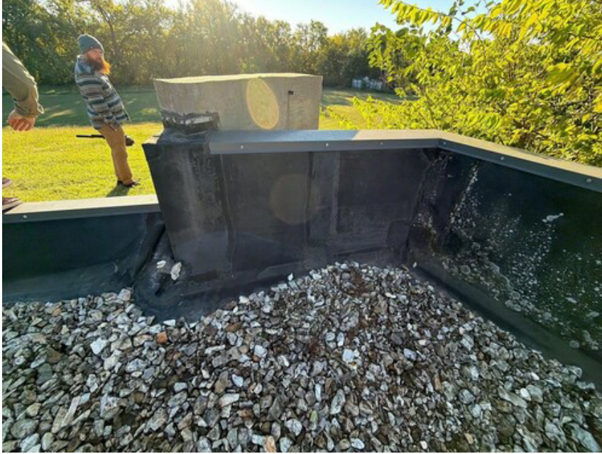
Area of hole into iso insulation tapered system, bottom left of picture
