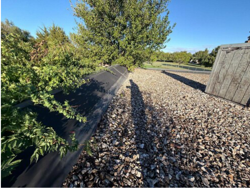
EDPM pulling away from side wall
