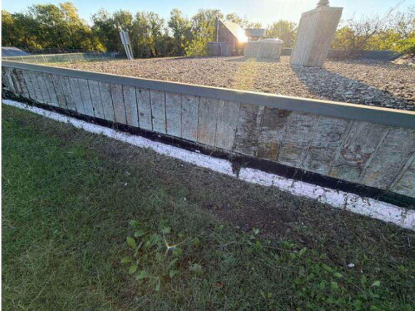
Major side wall deterioration
