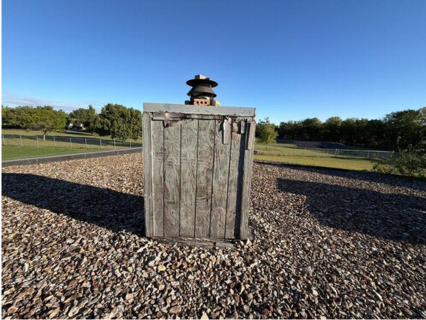
Major chimney deterioration
