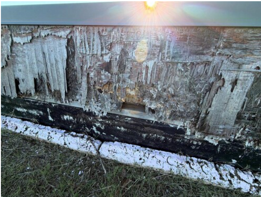
Major side wall deterioration
