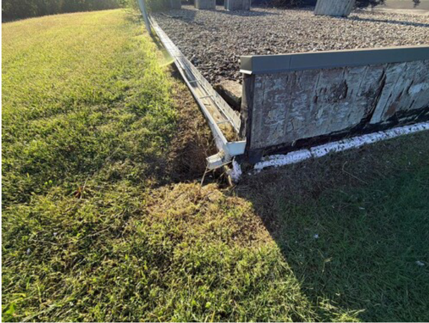
Major side wall deterioration and gutter downspouts dumping next to the hosue
