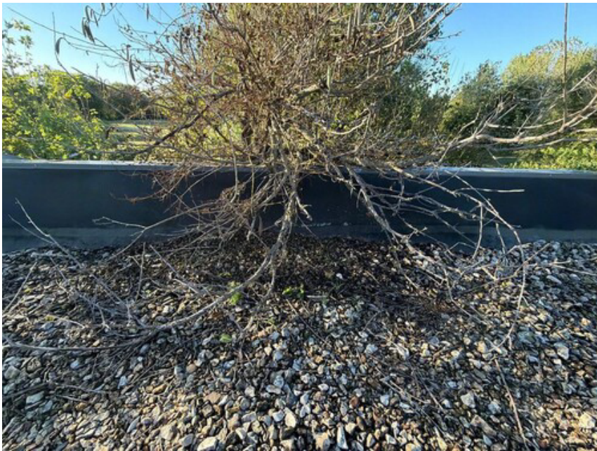
Over growth that may cause issues
