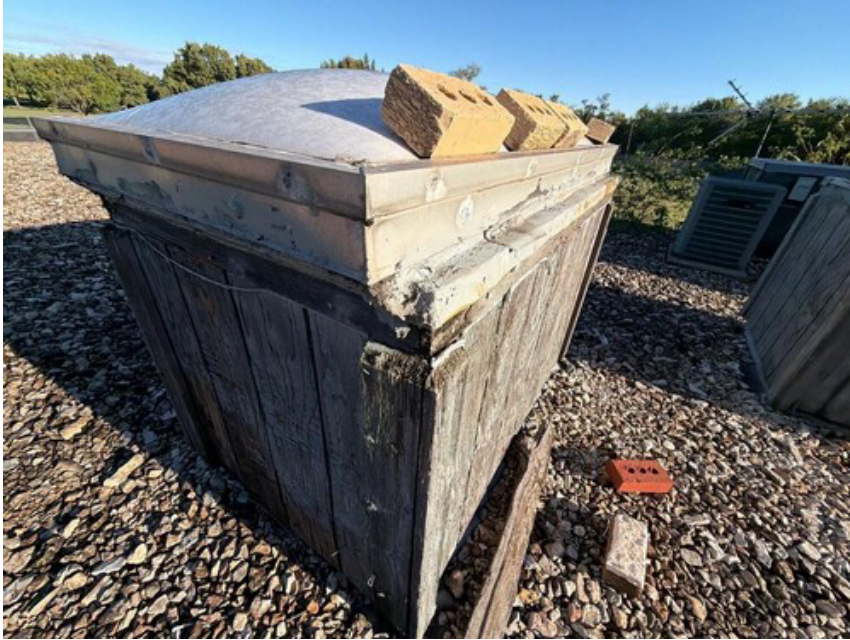
Skylight penetration, major deterioration
