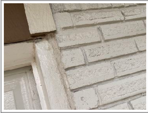
Sealed veneer separation on the southwest corner the garage
