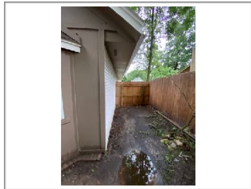
Standing water and missing down spout
