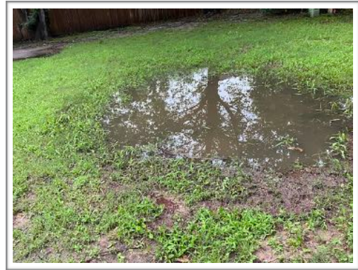
Standing water on the east side of the property
