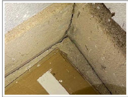
Stem wall crack and separation
