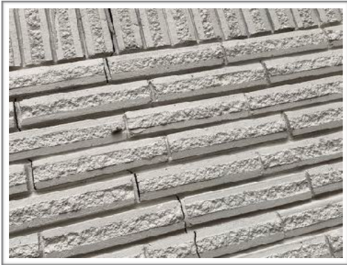
Exterior veneer crack on the south side of the garage
