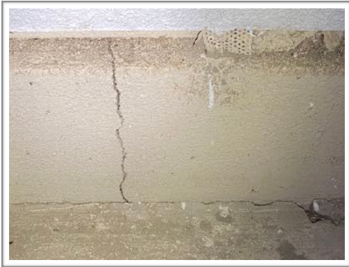
Stem wall crack
