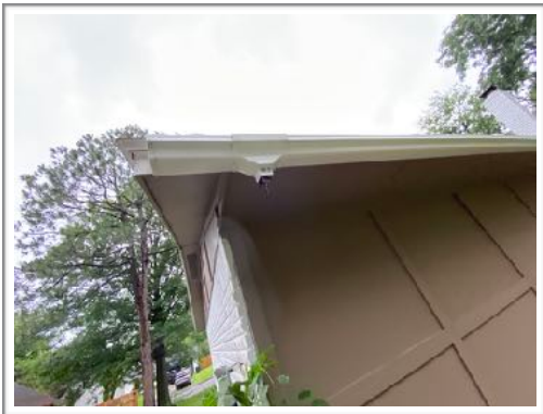
Missing down spout
